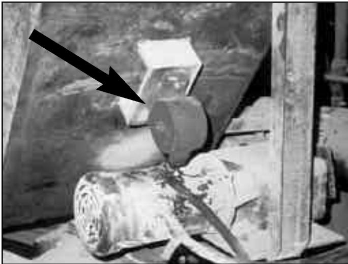
SILENT Turbine mounted to a fly ash chute to keep ash flowing.
